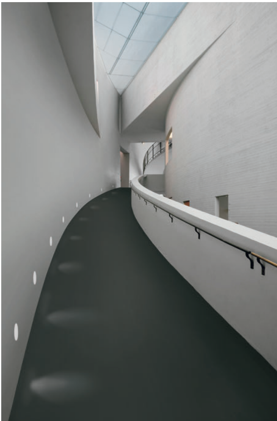
GYPSUM_WR RECESSED LIGHTS
